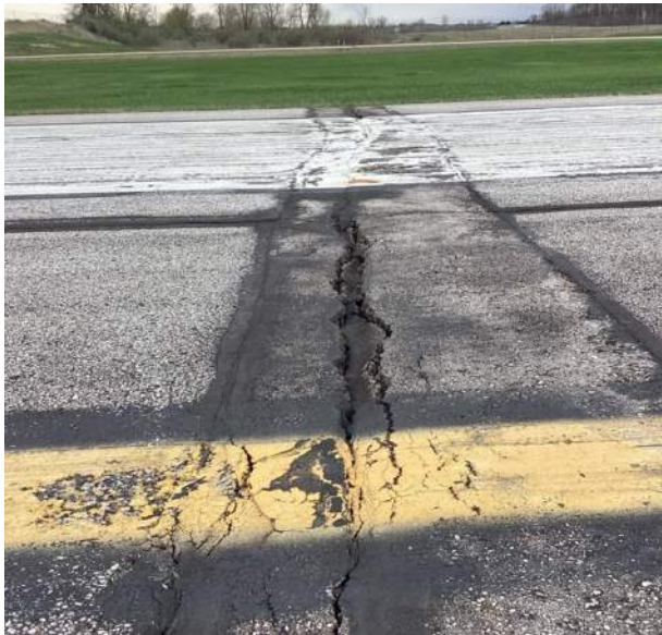
Figure 10 – Significant L&T Cracking on Runway
