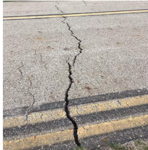
Figure 13 – L&T Cracking on Taxiway B
