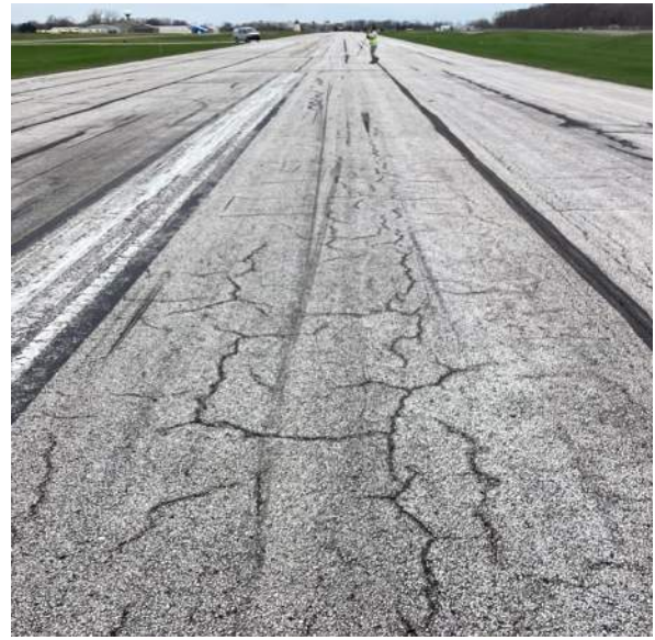
Figure 11 – Alligator & Block Cracking on Runway
