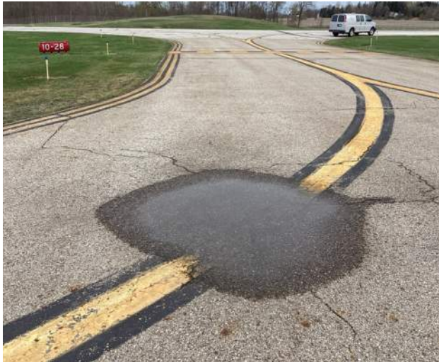
Figure 12 – Depression on Taxiway B
